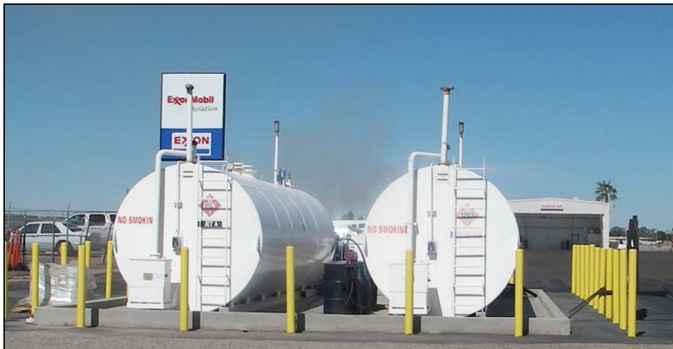
CareFlight Above-Ground Fuel Tanks
